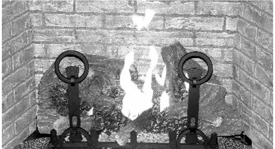
Figure 63 - Burner Flame Appearance
