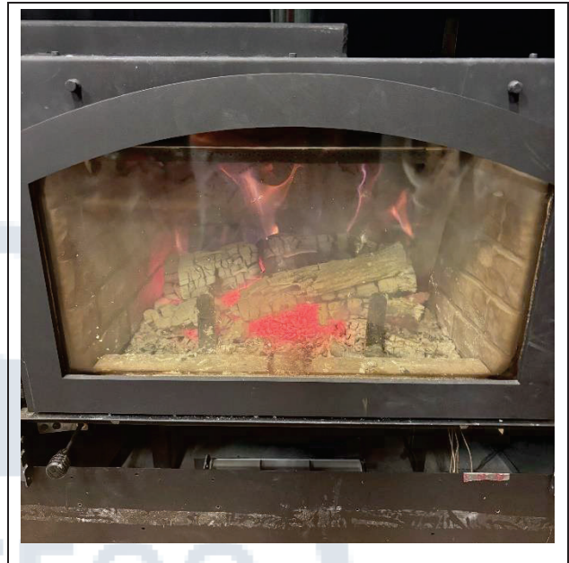
L2 Residual Fuel Loaded
